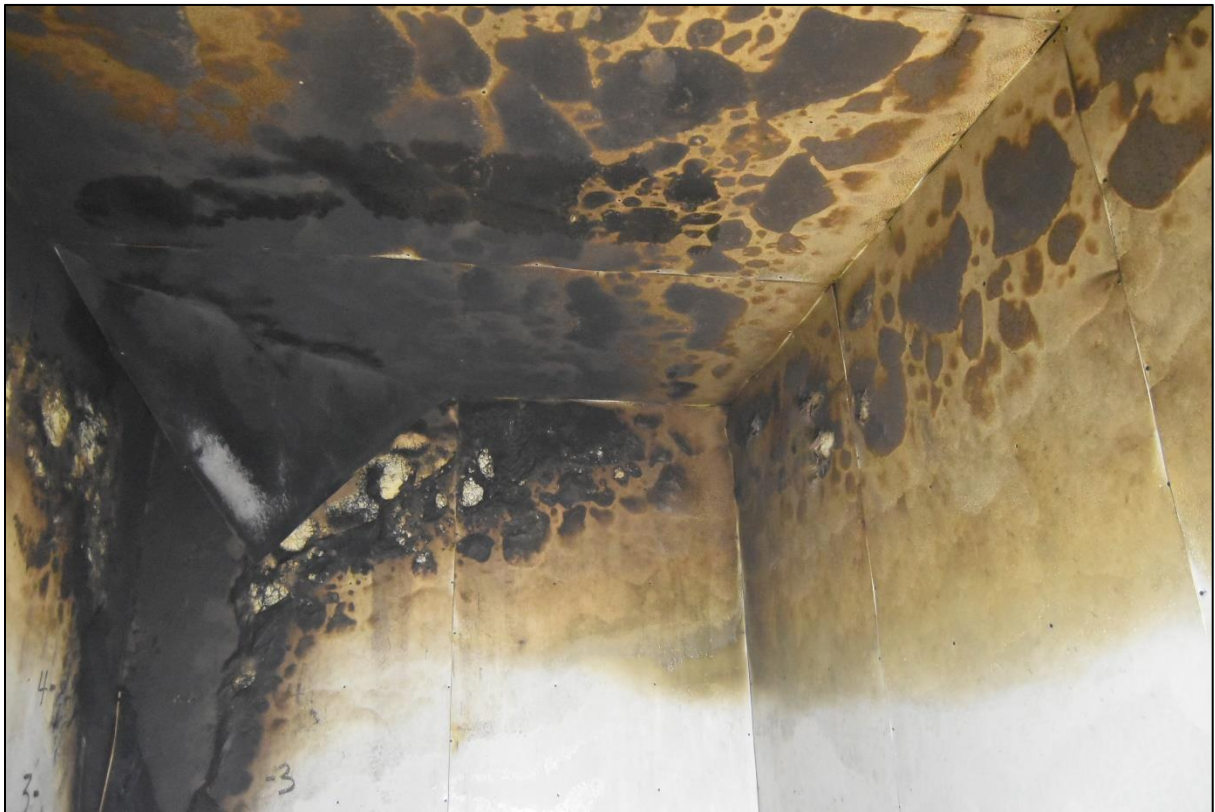
Figure A-10. Posttest View of Room Ceiling.
