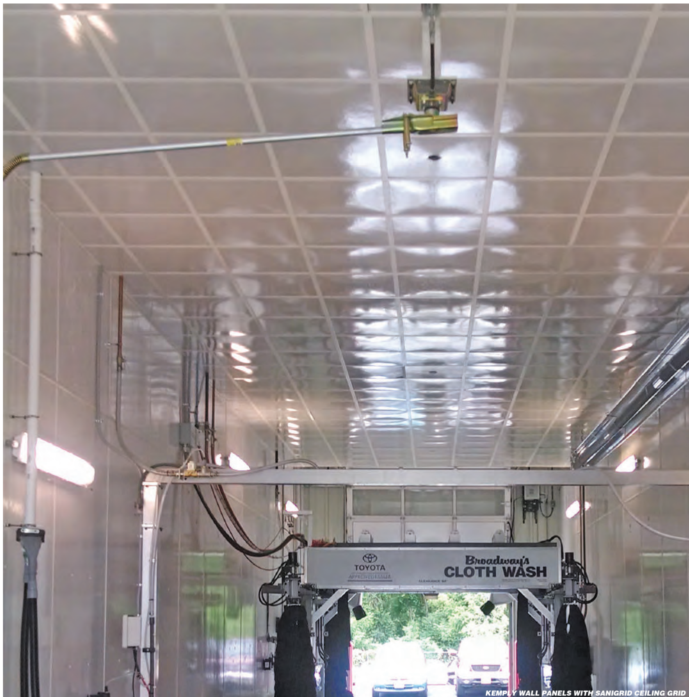
KEMPLY WALL PANELS WITH SANIGRID CEILING GRID FLUTED POLYPROPYLENE | EMBOSSED WHITE (85)
